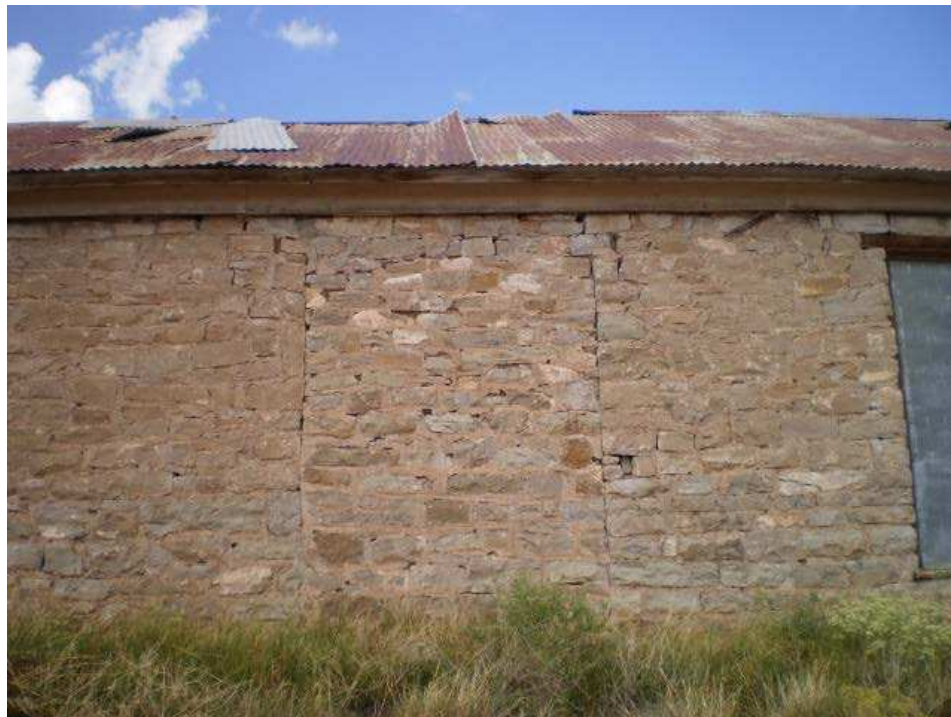
Figure 23 South View of 1893 Schoolhouse Showing Blocked Windows (Photo by Author, 2016)
